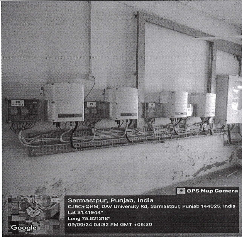
Solar Power Plant Inverter Room
